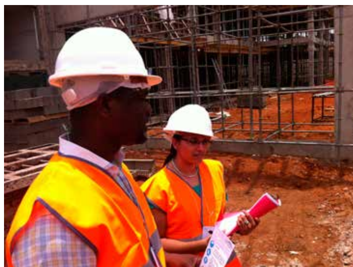
The HRIA team conducted a number of interviews with contractor's workers at the Nestlé factory construction site, Angola factory construction site, Angola
