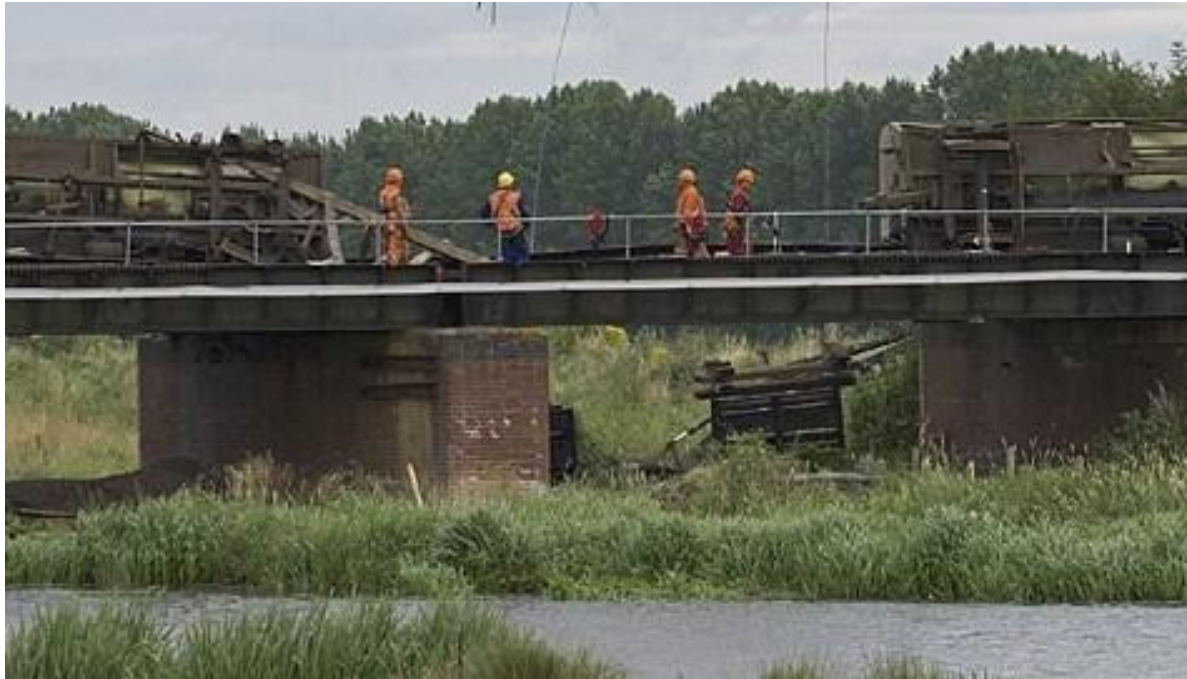
Figura 2 – The derailed wagons of freight train on Ely rail bridge [19]
