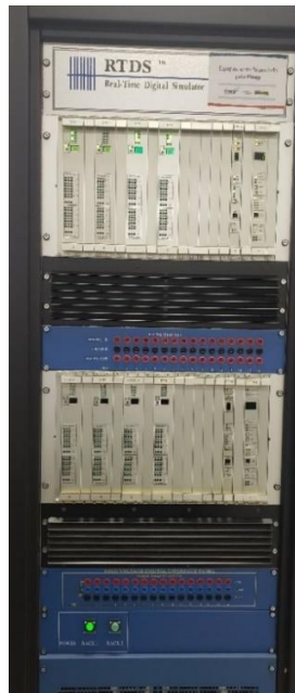
Figura 8 – Racks RTDS do LABSIM.
