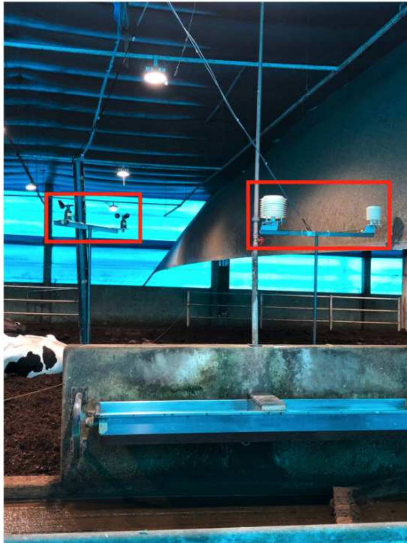
Figure 20-B - Sensors at Compost Barn.
